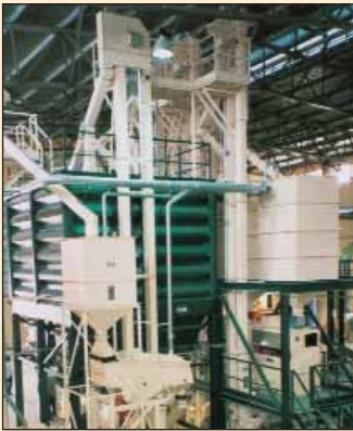
Nga Nam, Soc Trang Province, Vietnam. Integrated Paddy receiving, precleaning, drying and storage plant. Capacity 15 tph including 8 tph complete rice mill.
